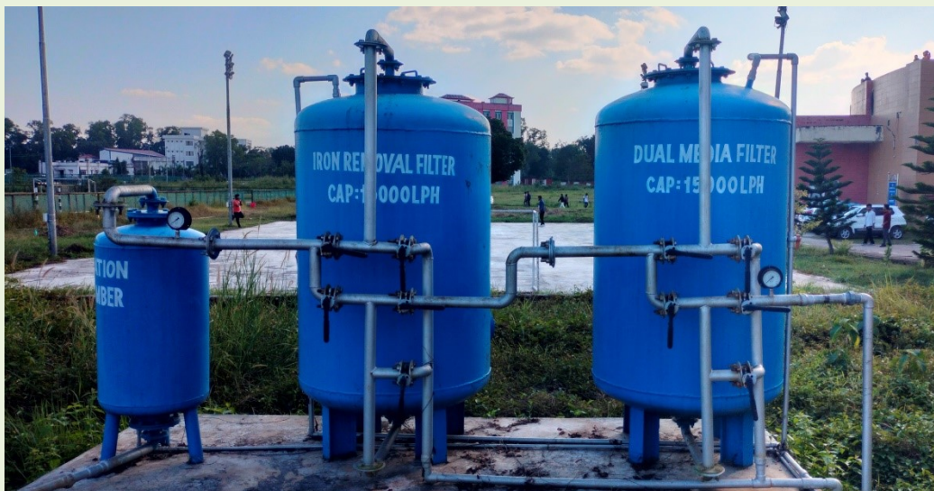
Fig 5: Water treatment facility
